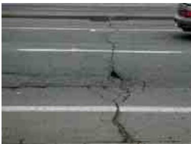
Figure 3c Severe Transverse Cracking
