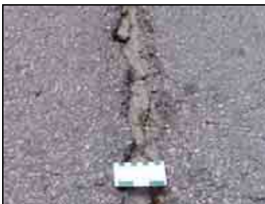
Figure 2.c Severe Longitudinal Cracking
