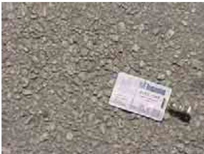
Figure 1a Slight Raveling
