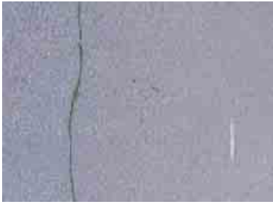
Figure 2a Slight Longitudinal Cracking
