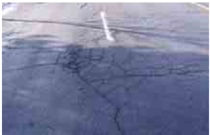
Figure 4b Moderate Alligator Cracking
