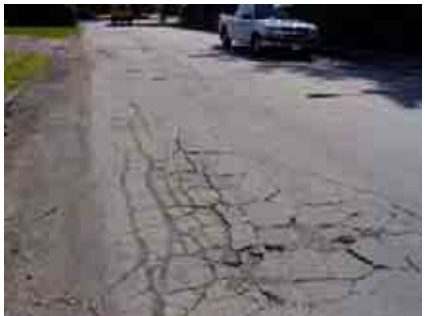
Figure 4c Severe Alligator Cracking
