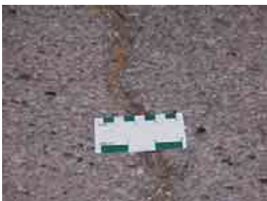
Figure 3b Moderate Transverse Cracking
