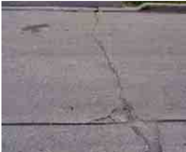
Figure 3a Slight Transverse Cracking
