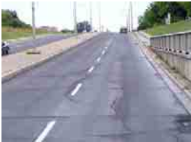
Figure 2.b Moderate Longitudinal Cracking
